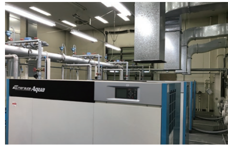
Oyama Factory: Consolidation and rationalization of air compressors
